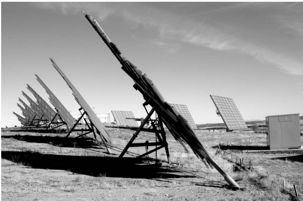
A geometric array of solar panels is part of the APS solar plant next to the Prescott Airport. They're pretty to look at, but the technology still has a long way to go before it's able to meet the Arizona Corporation Commission's 2015 renewable energy requirements. RIH photo/Erica Ryberg
